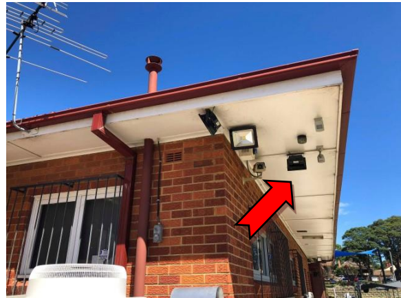
Photo 4. Exterior, main building, eaves – asbestos-containing fibre cement sheeting.
