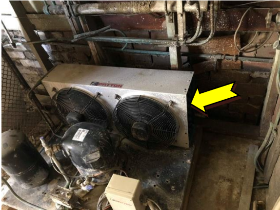
Photo 13. Exterior, back of house area, unknown refrigerant – suspected ODS-containing refrigerant gas.
