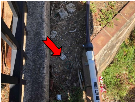
Photo 3. Exterior, south-eastern elevation, to ground surface – asbestos-containing fibre cement sheeting debris.
