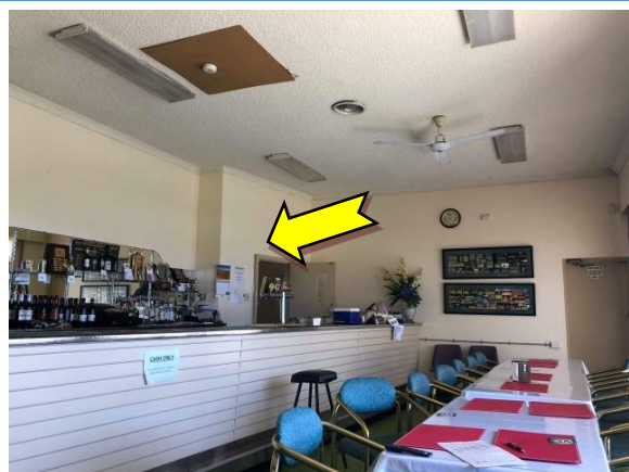
Photo 12. Interior, events room and bar area, walls – suspected lead-containing yellow upper paint system.
