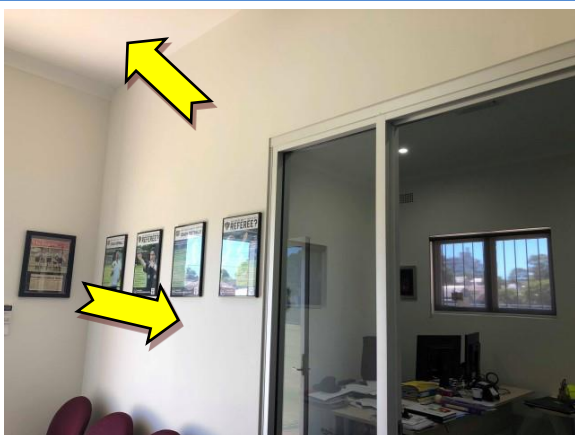
Photo 11. Interior, throughout, walls and ceiling – suspected lead-containing cream and white upper coloured paint systems.
