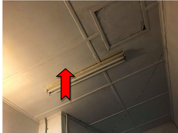
Photo 8. Interior, bar and kitchen toiler areas, ceiling – asbestos-containing fibre cement sheeting.
