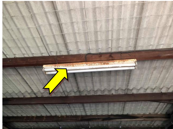
Photo 10. Interior, east elevation, shed, double tube fluorescent light fitting – suspected PCB-containing capacitor.
