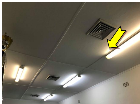
Photo 6. Interior, Canterbury soccer football office, main office, ceiling – asbestos-containing fibre cement sheeting.
